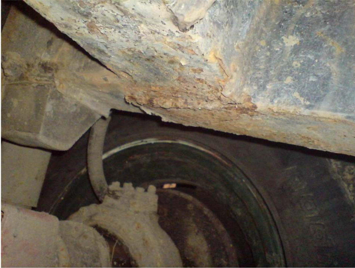
Just one example of an outrigger...the small holes were the start of it...it was shockingly thin...in the end I think every single outrigger was replaced:
