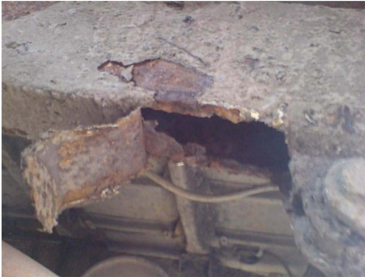
A quick inspection showed that the quality of the weld was, well, suspect....
